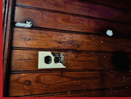
Broken and missing outlets
