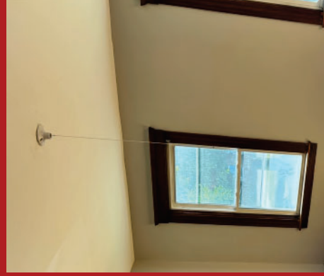
Pull string for living room lighting is not acceptable
